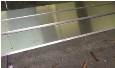
Surface area to be rubberized needs to be clean and free of grime or chemicals. Use ammonia based cleaner and paper towels.
